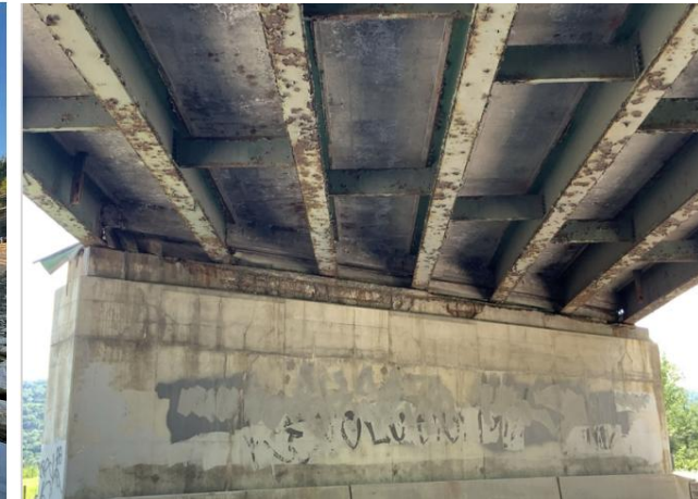
Aged Painted Girder with Peeling and Rust
